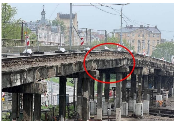
Figure 5. Deformation of the overpass span beam.
