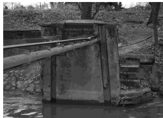
Figure 5. The fortress weir XI ( Nadelwehr - St. W. XI ) in a state of major disrepair, 2012 (Source: photo by the author, 2012)
