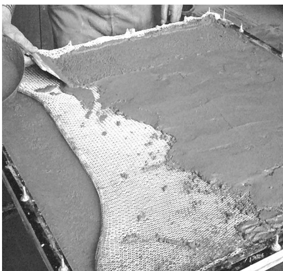
Figure 2. Concrete shell fabrication reinforced by three layers of knitted glass fiber fabric
